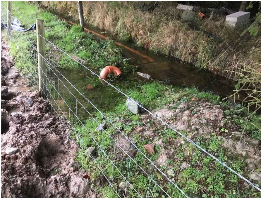
Figure 3 View of ponding at drainage outfall
